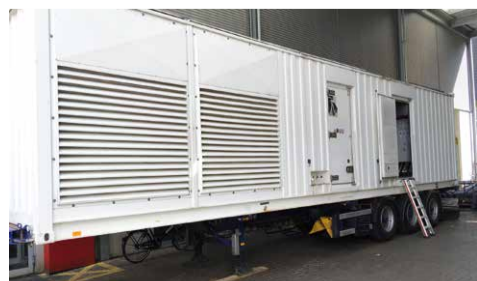
Aerzen Rental contributed a 1.2 megawatt diesel generator for the function test.
