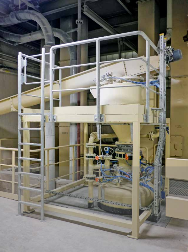
ISS Schüttguttechnik has planned and realised the new stucco supply together with Knauf Engineering.
