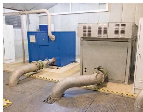
New meets old: the old-fashioned blowers now serve as redundancy and standby for peak loads.
