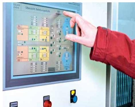
The blower technology can be operated on site via a touch panel.
