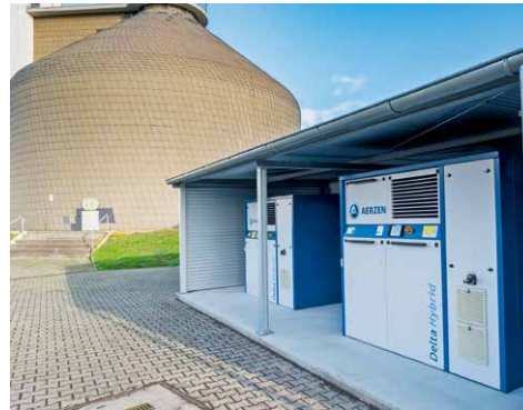
Two Delta Hybrid machines are placed under a protective roof outside the wastewater treatment plant.
