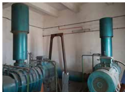
The production line at the cement plant was in a disastrous condition.
