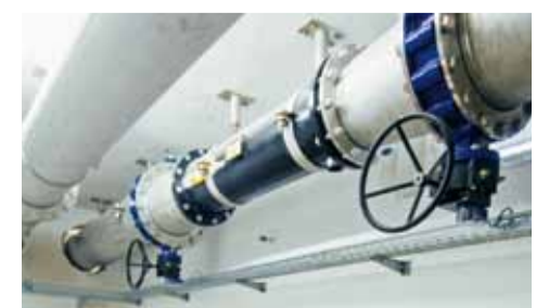
A pipe bundle heat exchanger recovers heat in the blower air.
