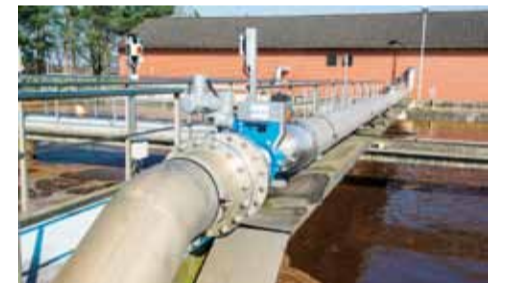
With diaphragm regulating valves and modified speed the air introduction into the tanks is controlled.
