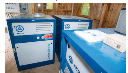
Three energetically optimised AERZEN Delta Blowers play an essential role in heat recovery at the Wertach wastewater treatment plant.
