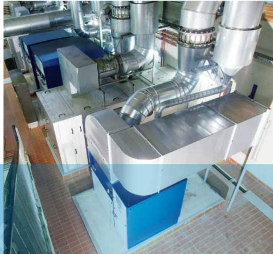
View onto the compressor station with turbo compressor from AERZEN, an old turbo compressor, two rotary lobe compressors Delta Hybrid from AERZEN and two further old turbo compressors (from front)
