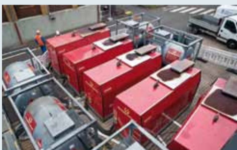
View of the diesel motors and the reservoirs for diesel fuel.
