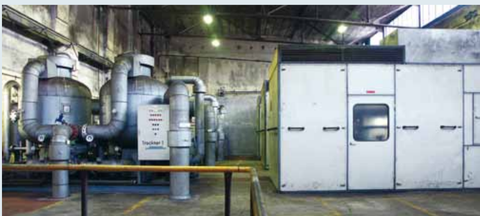
The central compressed-air-station of Brikettfabrik Wachtberg: - on the right three enclosed Aerzen Screw Compressors: - on the left three adsorption dryers.
