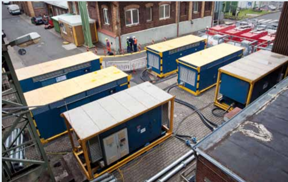
Six Aerzen Screw Compressors for external compressed-air emergency supply, as well as emergency-units and diesel tanks were installed on the paved courtyard in front of the central compressed-air station.
