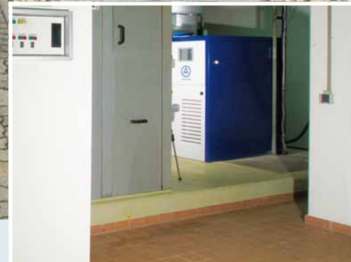
Besides a positive displacement blower series DELTA BLOWER, which extracts exhaust air and feeds it into the aeration basins, wastewater treatment plant Arnsberg-Wildshausen also has a new Aerzen turbo blower in the central compressed air station.
